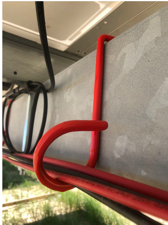
Figure 3: Torque Tube Hanger Supporting String Conductors
